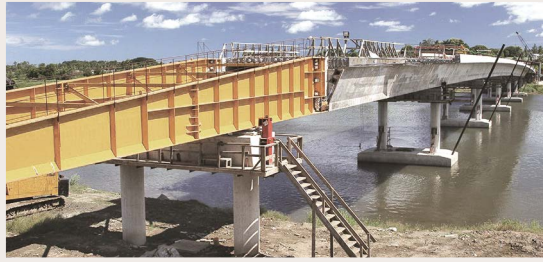
The 40 tonne steel bridge box girder casting mould fabricated by FSHIL, which was used in the construction of the new Rewa bridge completed in 2006.
